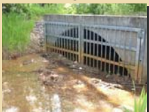
Fig. 2. Screen culvert near airport clogged with debris.
